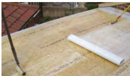
A polyester roller is used to apply the resin to the Reinforcement Mat. Cure It Roofing Resin is applied to the deck before the Reinforcement Mat is laid on the roof.
